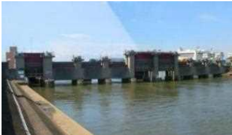
An example of coastal gate designed to allow easy renovation for the increase in future sea level rise
